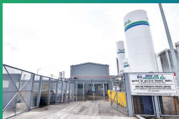
Our first on-site Nitrogen Installation for Solar PV Cell Industry Commissioned for First Solar
